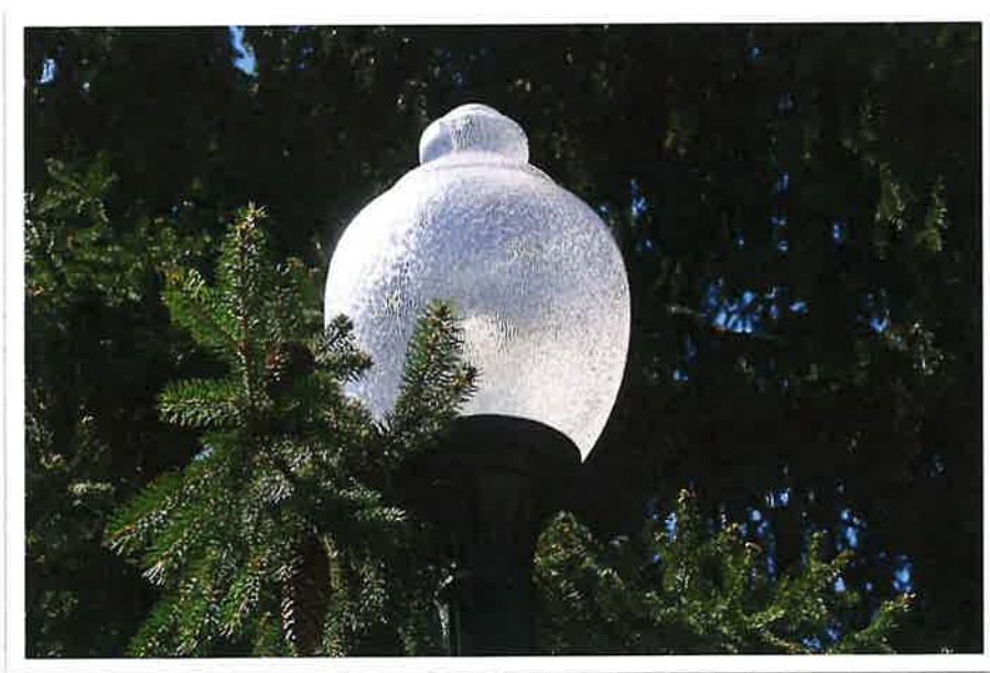
Photograph 10: Typical view of pole light
