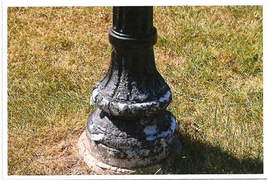
Photograph 15: Typical view of street sign
