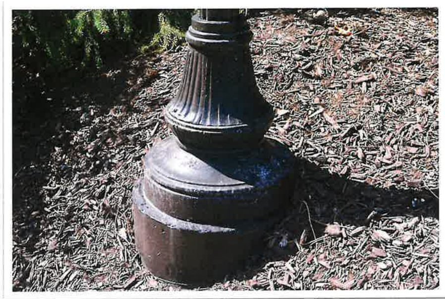
Photograph 9: Typical view of pole light
